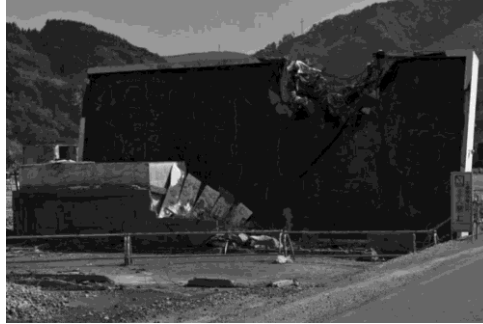
Fig. 23. Serious damage observed on the roof of Building E overturned probably due to collision of Building D [3]
